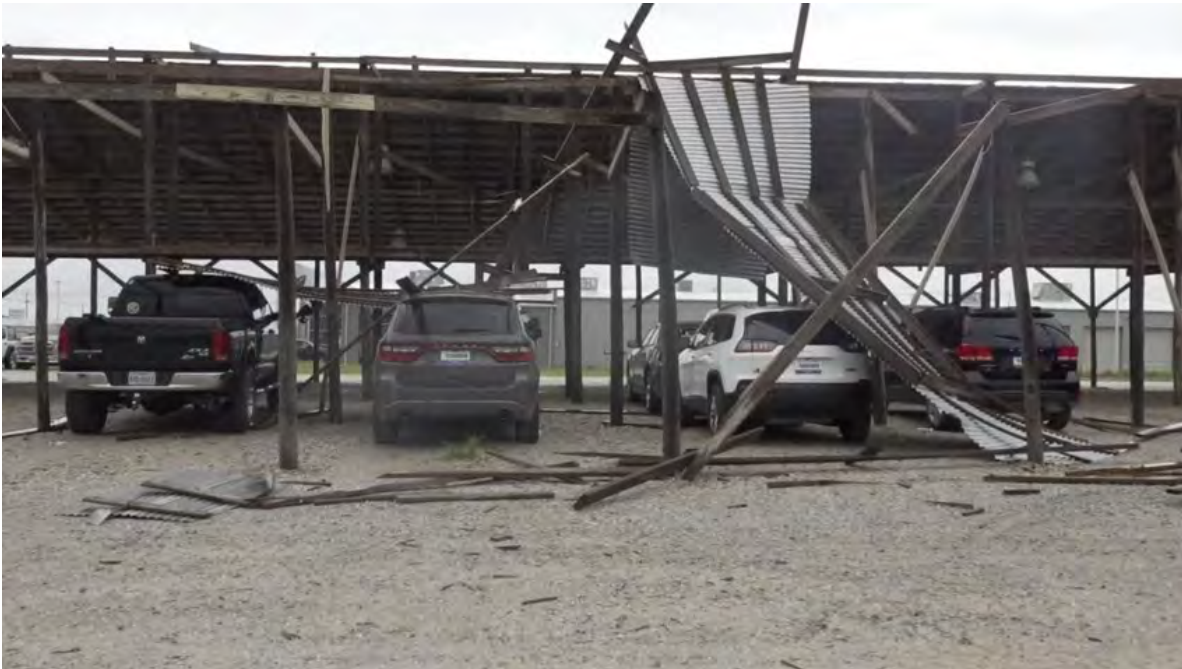
Figure 9-2: Wind damages to dealership. (Source: FOX West Texas)
